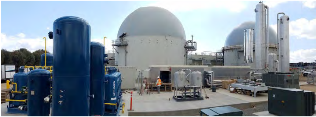
CR&R Anaerobic Digestion of MSW to RNG
