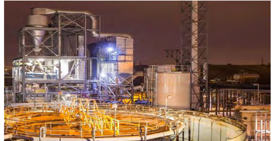
Rialto Bioenergy/Anaergia Anaerobic Digestion & Pyrolysis of MSW and Biosolids to RNG
