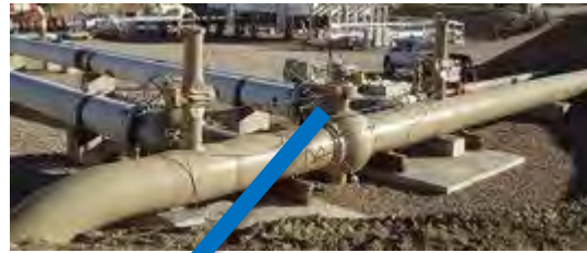
CNG/RNG Pipe Line Located at the Locomotive Refueling Yard
